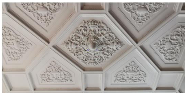
Fig. 11: Stucco ceiling of the room with a terrace. Photograph courtesy of Helder Carita.
